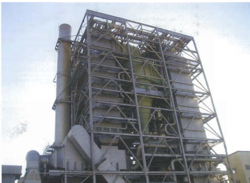
View of circulating fluidized bed boiler
