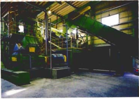
Plastic waste that has previously been crushed into the form of flakes is further compressed into high-density flakes in this reducer. This marks the final stage of the pretreatment process.
