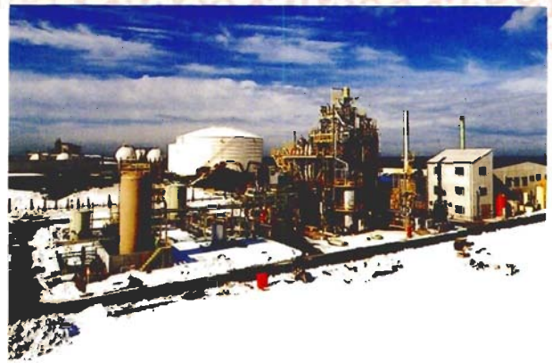
This overall view of the Niigata Plastics Liquefaction Center shows the plant for the pretreatment process in the background on the right and the plant for the liquefaction process on the left. This facility can treat 6,000 metric tons of plastic waste annually.
