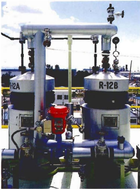
In these catalyst vessels, the chlorine fraction is removed from the oil that has been formed by pyrolysis. Terephthalic acids are decomposed and other small amounts of constituents are regulated.
