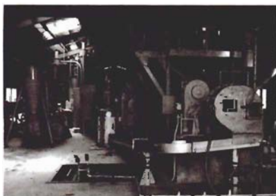
Experimental facility in Funabashi City in Chiba Prefecture for recovering sorted plastic waste through a melting process
