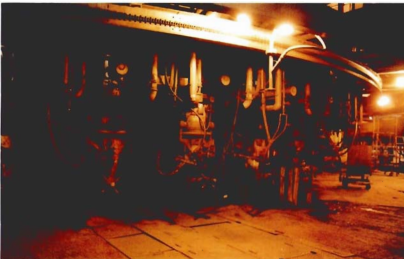
Tuyeres around the lower part of blast furnace
